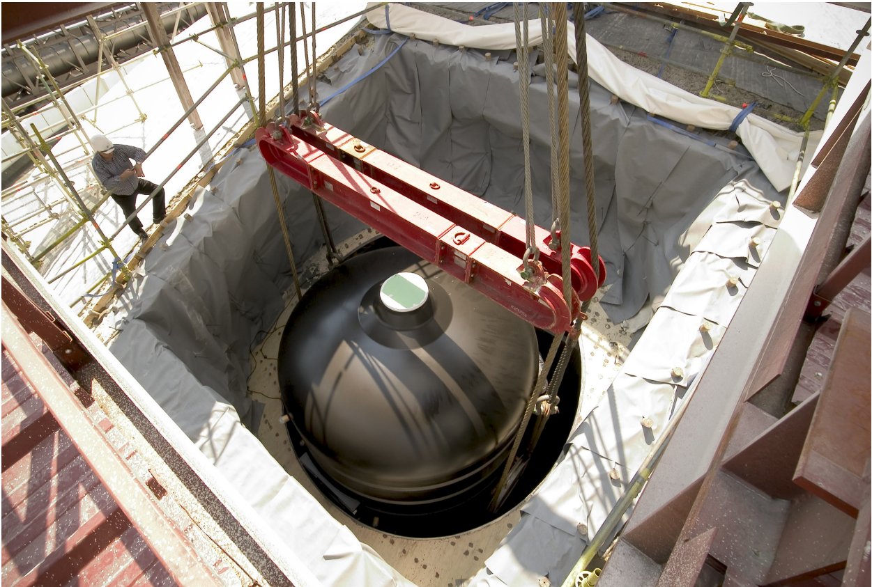
Figure 1.5 – Steam generator replacement through a hole cut into the containment at the Belgian nuclear power plant Doel 2, 2004. (© electrabel)
