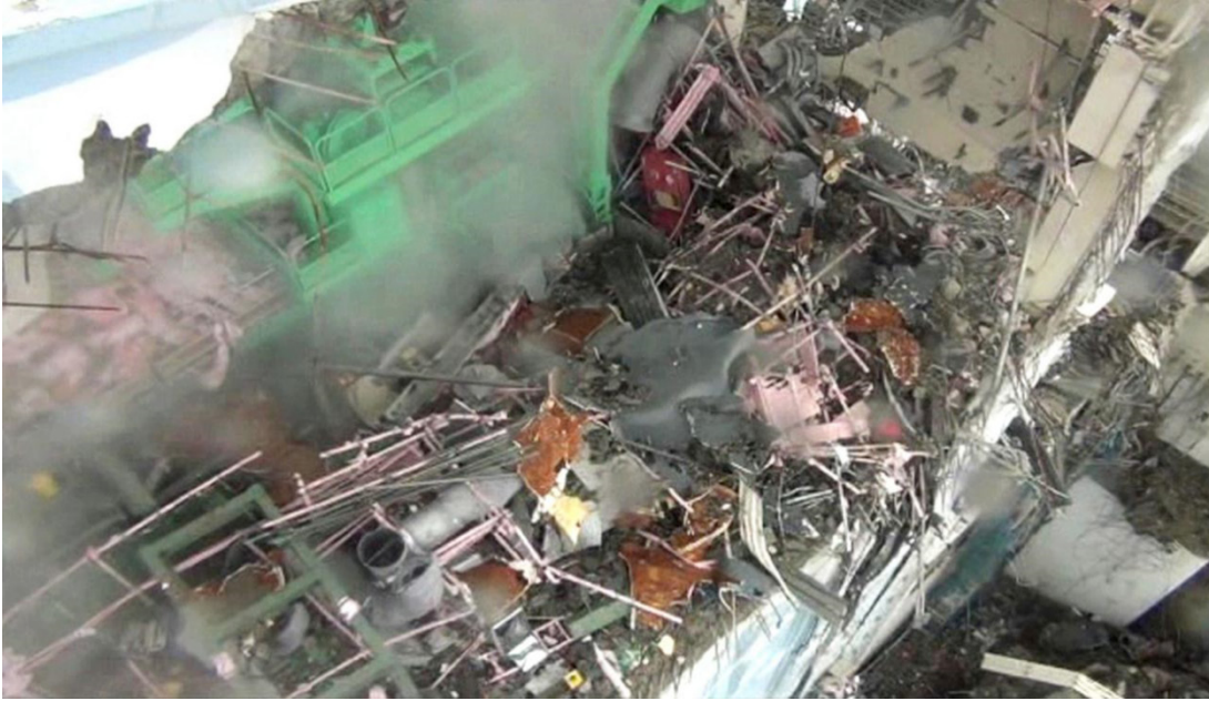
Figure 1.11 – Debris in the spent fuel pool of Fukushima-Daiichi 4 after the hydrogen explosion, with steam rising. Source: TEPCO.
